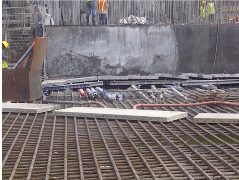
Fig. 3 – Honeycombing in stripped block of New Panama Canal
